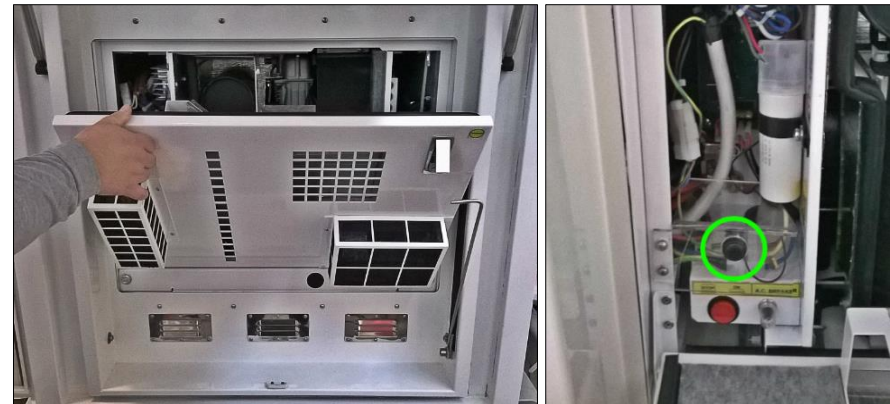
Fig. 19 – Fuel filter cleaning
