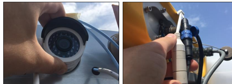
Fig. 4 – Pointing Camera - Camera Supply and Ethernet cables
