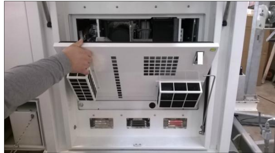
Fig. 14 – Generator rotating panel
