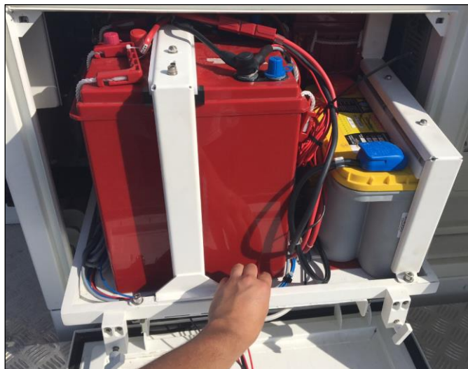
Fig. 9 – Sliding batteries drawer
