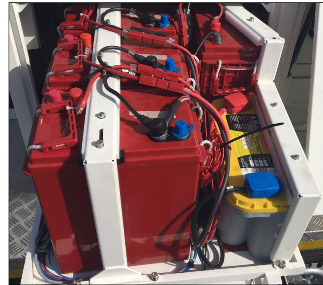
Fig. 10 – ArcSAR Batteries on the drawer
