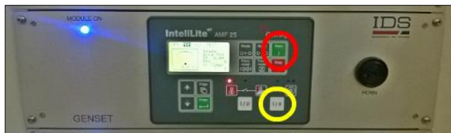
Fig. 26 – AMF25 control panel
